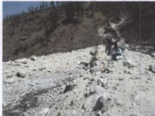
Photo: Land slide requiring treatment
